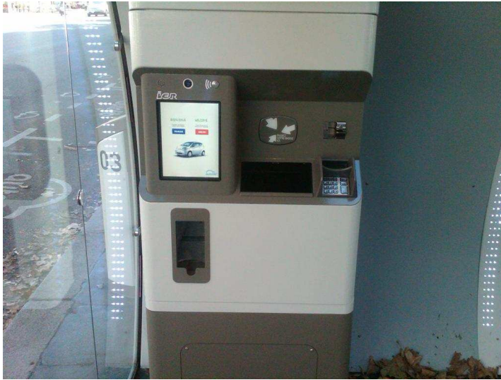
A1 17 - AutoLIB Charge Point Payment System in Paris
