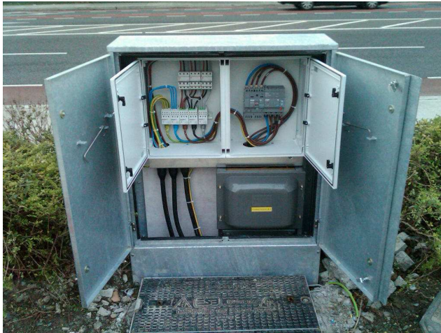
Figure 4.10 - Internals of Multiple Charge Post Interface Pillar
