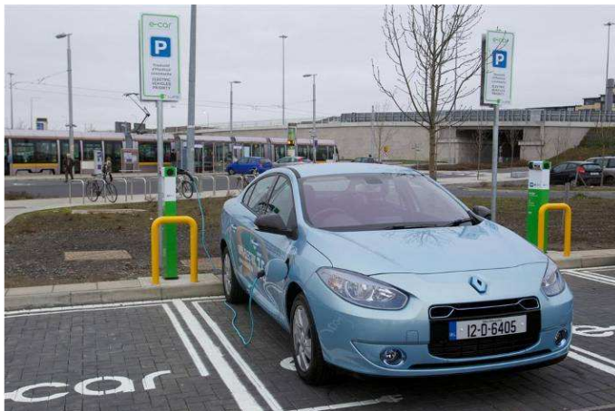
Figure 4.5 - Multiple Charge Point in Park & Ride Facility in Ireland
