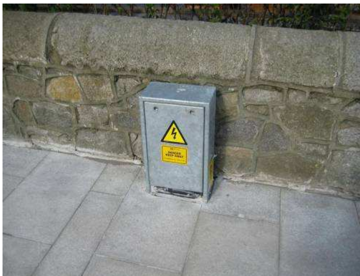
Figure 4.7 - Single Charge Post Interface Pillar
