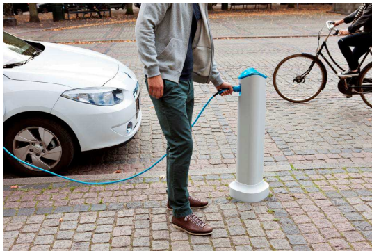
Figure 4.3 - Charge Point Installed on Cobblestone Pathway in Copenhagen
