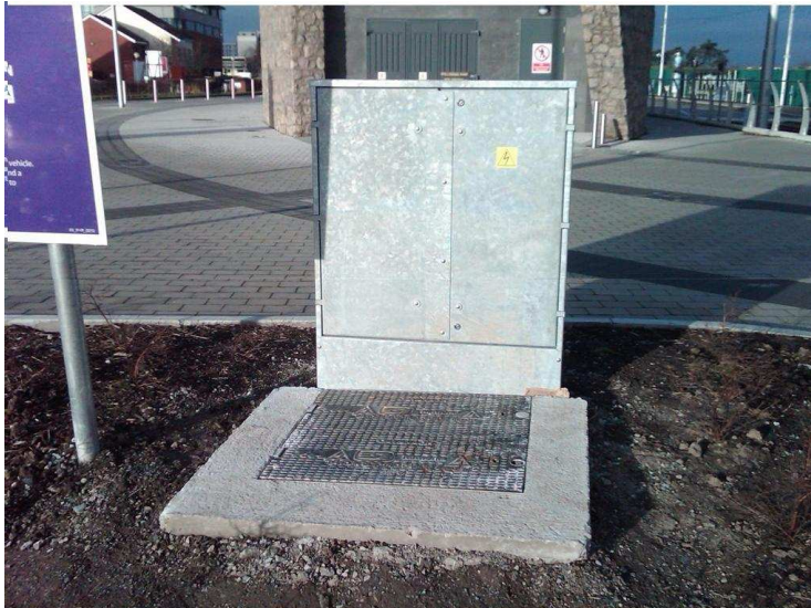
Figure 4.9 - Multiple Charge Post Interface Pillar
