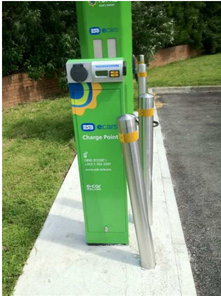
Figure 4.14 - Stainless Steel Bollards Damaged by Vehicle
