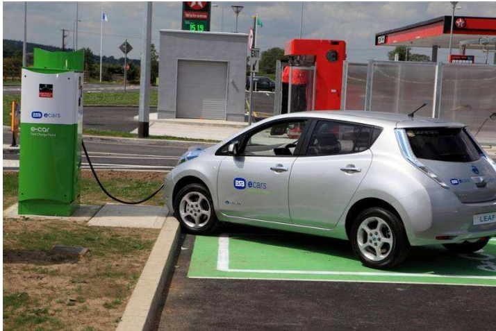
Figure 4.6 - DC Charge Point in Fuel Service Station
