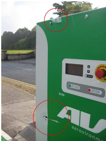
Figure 4.15 - Damaged DC Charge Point
