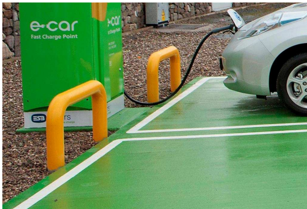
Figure 4.13 - Bollards Protecting DC Charge Point
