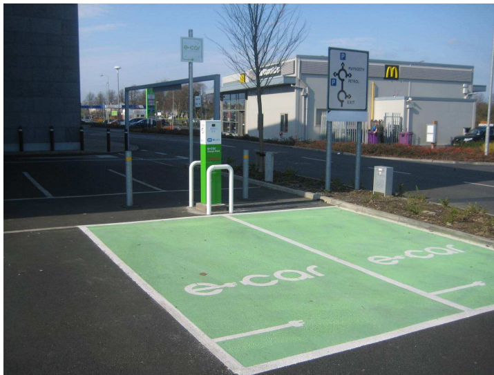
Figure 4.1 - Charge Point in Shopping Centre Carpark
