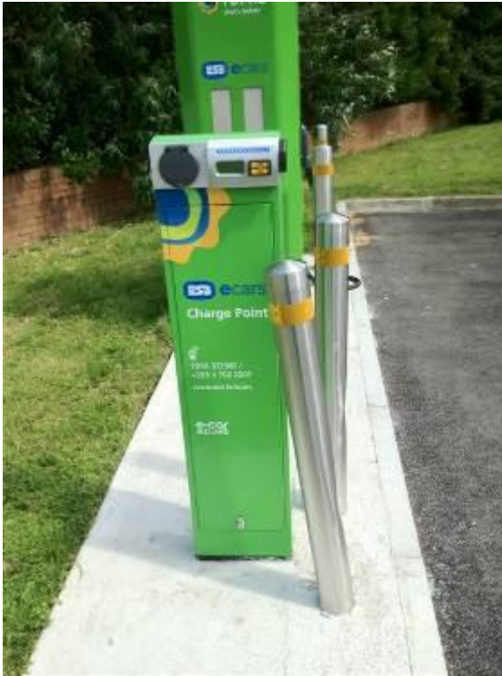
Figure 4.15 - Stainless Steel Bollards Damaged by Vehicle
