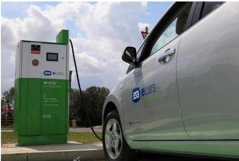
Figure 2.3 - DC Charge Point
