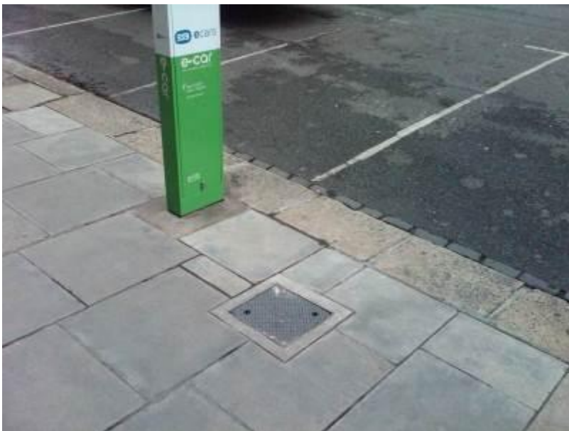
Figure 4.12 - Underground Vault in Ireland
