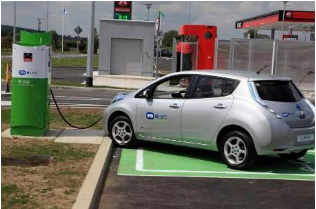
Figure 4.6 - DC Charge Point in Fuel Service Station
