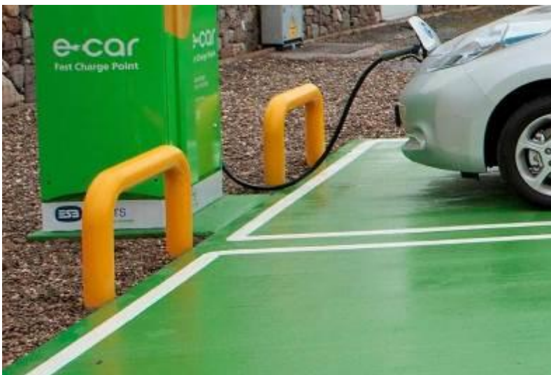
Figure 4.14 - Bollards Protecting DC Charge Point
