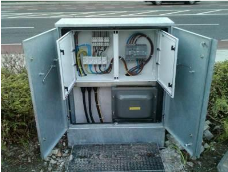
Figure 4.11 - Internals of Multiple Charge Post Interface Pillar
