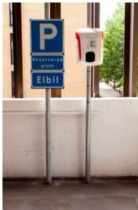
A1 3 - Charge Point in Park House in Malmo 3
