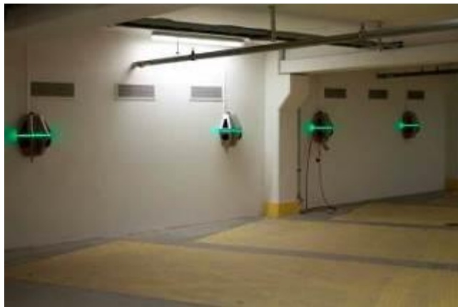
A1 2 - Charge Point in Park House in Malmo 2
