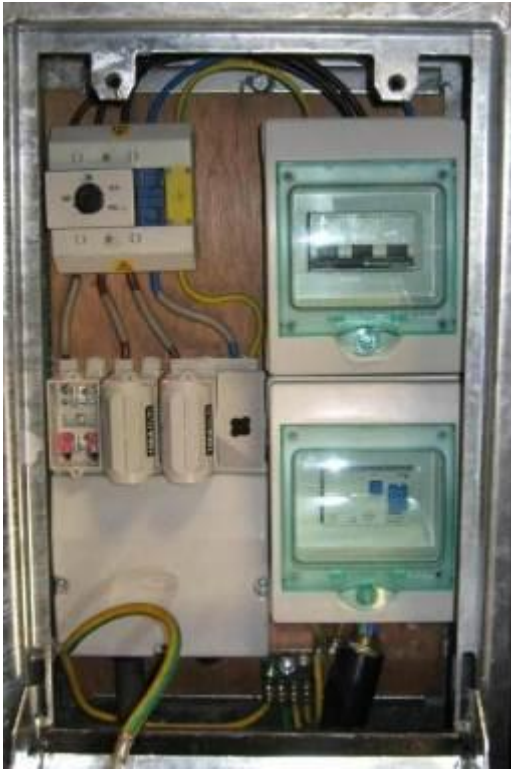
Figure 4.9 - Internals of Single Charge Post Interface Pillar
