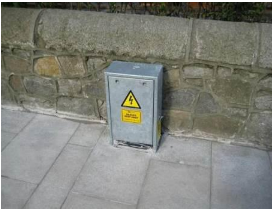
Figure 4.8 - Single Charge Post Interface Pillar
