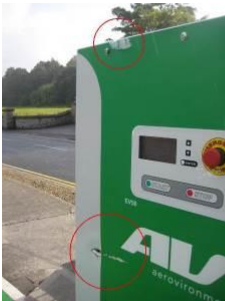
Figure 4.16 - Damaged DC Charge Point
