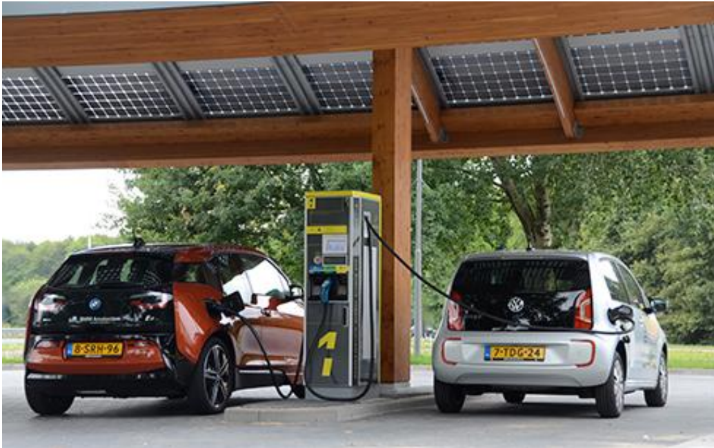
Figure 2.7 – Fastned installation in the Netherlands
