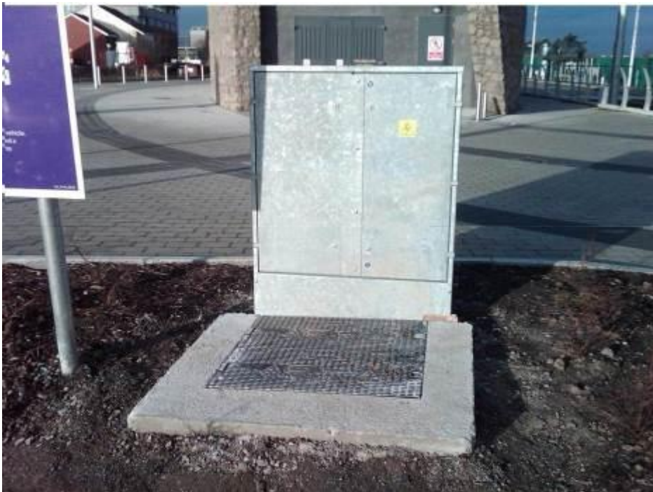
Figure 4.10 - Multiple Charge Post Interface Pillar
