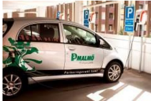
A1 1 - Charge Point in Park House in Malmo 1
