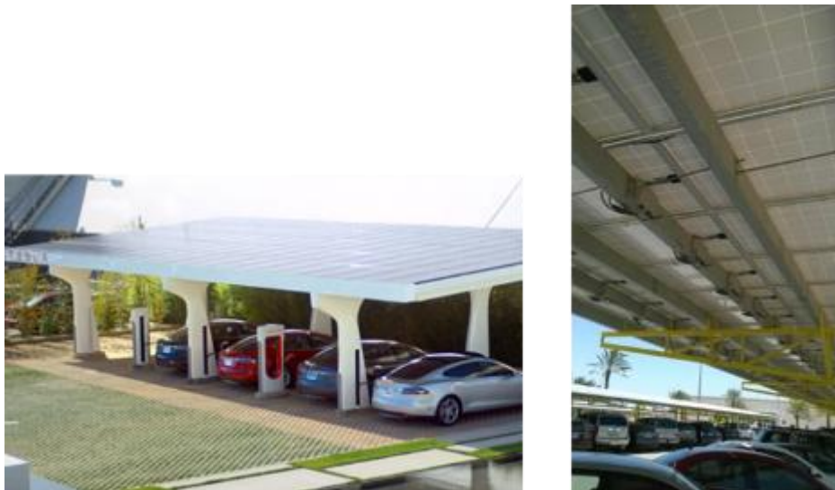
Figure 2.6 – Tesla Solar Charging – California ~30 kW Solar and a Solar car park in Bahrain
