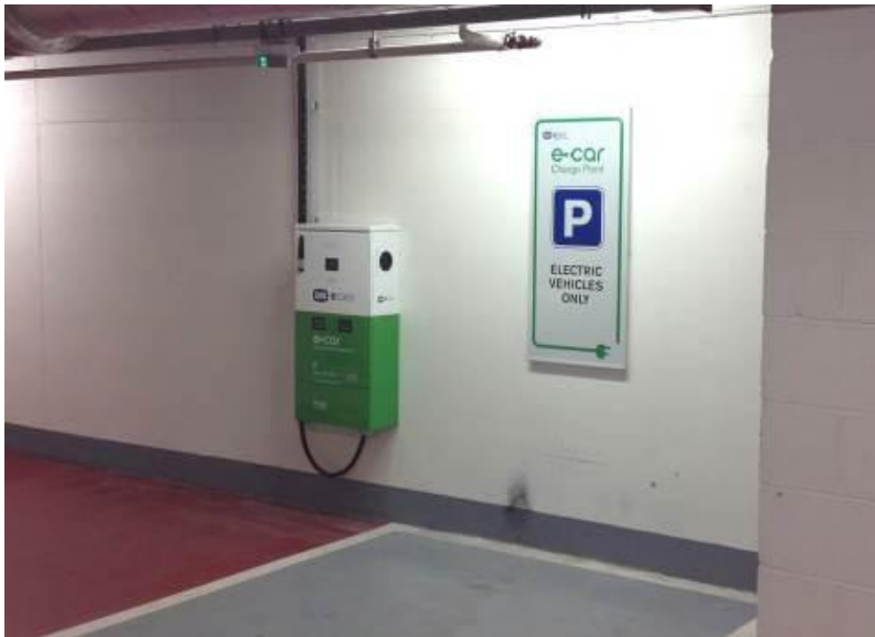
Figure 4.7 – Charge Point in Shopping Centre Carpark
