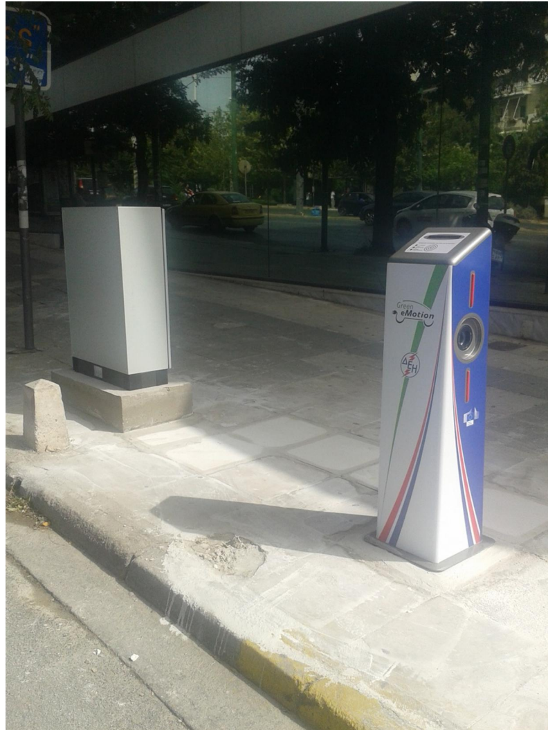
Figure 2.3: DSO external meter next to a charging station.
