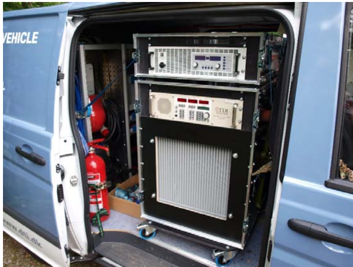
Figure 3.3.1: Mobile load bank unit in the battery service vehicle
